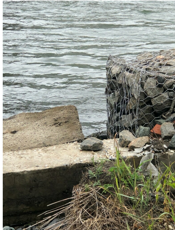
The crumbling seawall.
