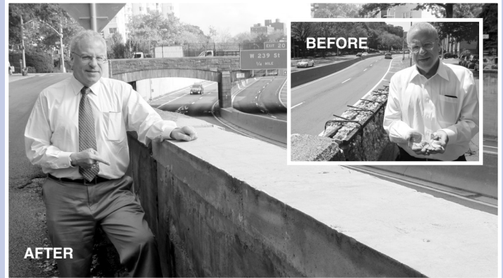
After raising concerns about the deteriorating retaining wall bordering the Henry Hudson Parkway at the 232nd Street exit, the NYS Department of Transportation has responded to the request by Assemblyman Dinowitz and has made significant repairs.
