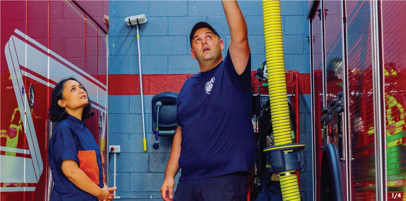
Photo: Getting a tour of a ventilation system at the Glasco Fire Company we helped secure a $100,000 grant for. The system reduces exposure to carcinogenic diesel contaminants by preventing particles from accumulating on equipment and turnout gear. The New York Health Act would provide comprehensive health- and long-term care to every New York resident, including volunteer firefighters who put their health at risk all year round.
